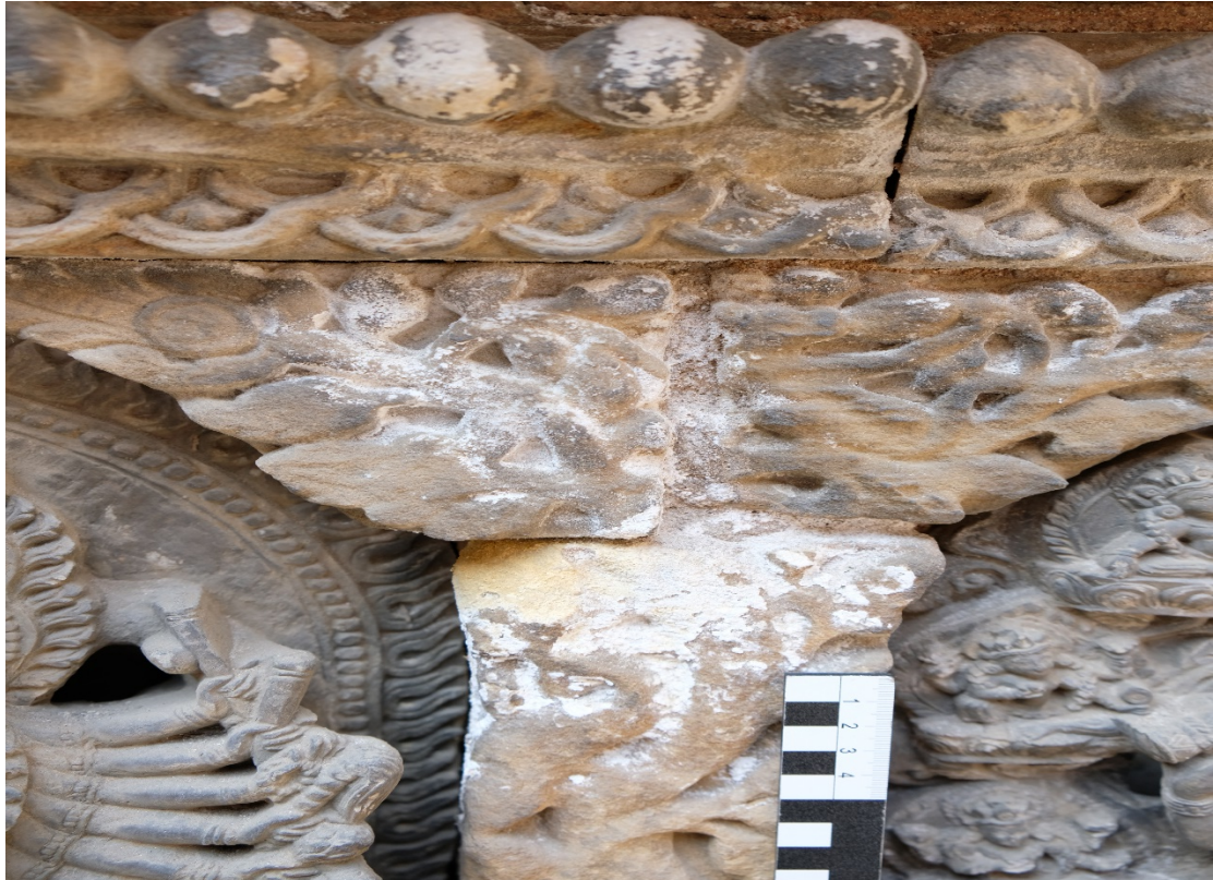
Fig: 2: Problem of salt efflorescence in Tusha Hiti, Royal Palace.
