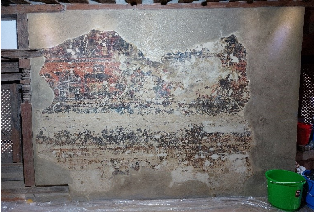
Fig: 7: Wall painting after conservation treatment.
